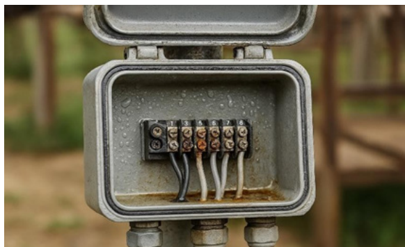
Figure 1: Moisture ingress and condensation inside field junction box leading to terminal degradation
