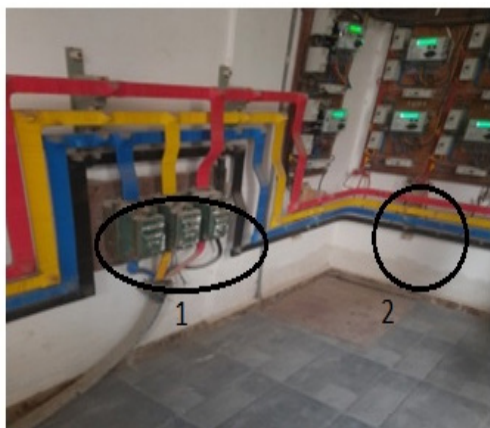
circle 1, Main supply from to Fuse Figure 1 Circle 2, Open busbar with PVC Tape.
